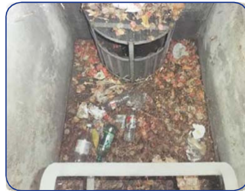
The City cleans and inspects 250 trash capture devices quarterly, removing 40 cubic yards of debris annually.
