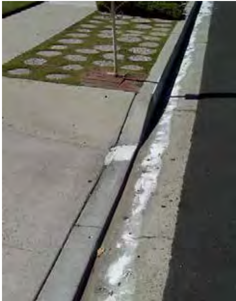
Evidence of an illicit discharge
